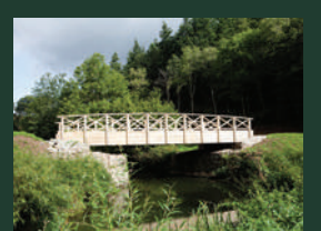
Joiner's Bridge Stop to take a photo on our glorious handcrafted green oak bridge
